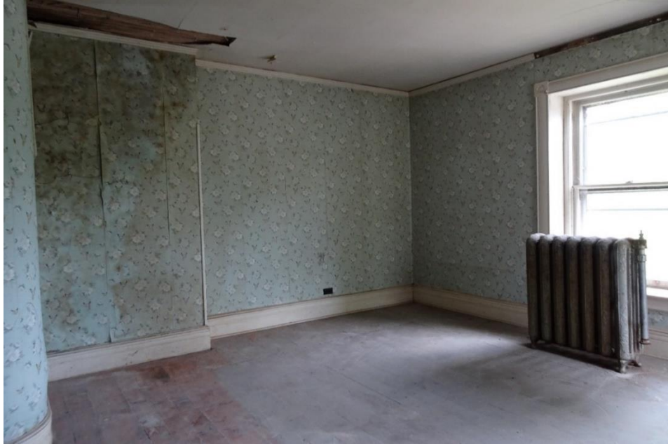
Fig.40: Water infiltration Damage, Second Floor, Room 203
