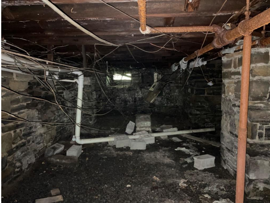
Fig.50: Pipes and Electricity Wires on the Basement
